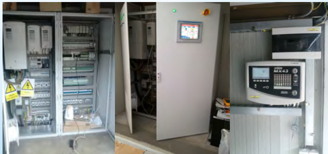
Control system of package
